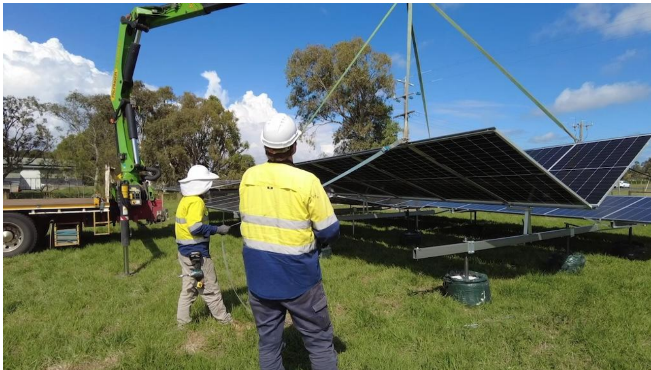
Solpod on ballast blocks
